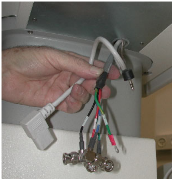
Figure 8-153 Color Printer Cables through Metal Bottom Cover Slot
